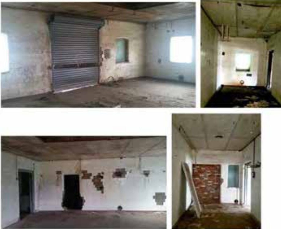
Figure D9. Area H (left) Looking north. Showing the original segmental arched window openings in the north elevation and the square window opening in the east elevation, all with architraves of curved white glazed tiles and white glazed tiles on the walls, and red-brown hexagon tiles on the floor. The roller door is a later alteration. Area I (right) . Looking east to the square window opening, and west to the bricked up opening, with walls clad in white glazed tiles. Note the ceilings may be asbestos cement sheeting. Source. Andrew Martin 2017.
