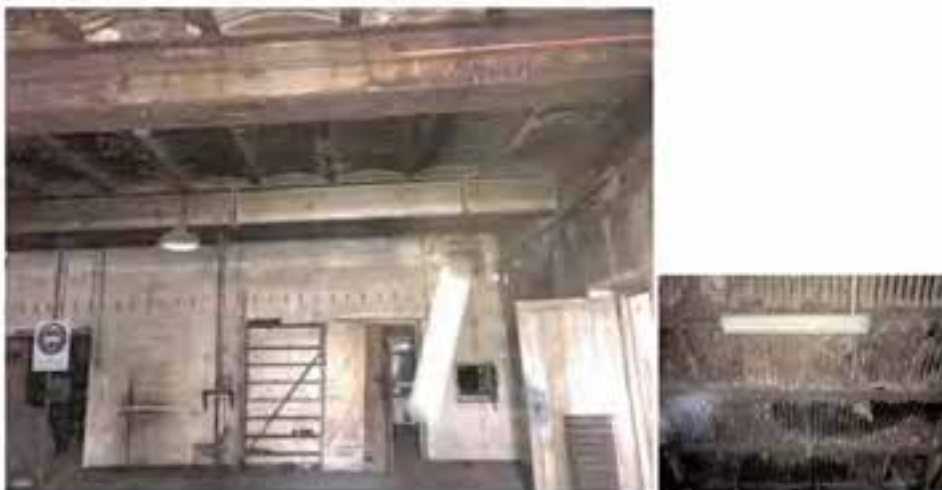
Figure D5. Blue Area A. View looking south towards the doorways into Areas B and C. The door on the right goes into Area F. Note all the walls are lined with glazed white tiles (now dirty) as are the architraves and reveals, the floor is lined with matt finish hexagon shaped brown-red tiles and the ceiling appears to be comprised of wrought iron joists supporting arched, deep-gauge (?) corrugated iron. The roof appears to be supporting a concrete floor. The method of construction is now rare, and appears to be similar to that used in the Queens Warehouse, Melbourne and described by Miles Lewis as 'Lysaght's Galvanized Tinned Iron 20 Gauge [sic]; Heavy Weight ... equal to sample'; and 'Traegerwellblech'. "In 1902 Lysaght's Metal Trades Reference listed 'weight-bearing'
