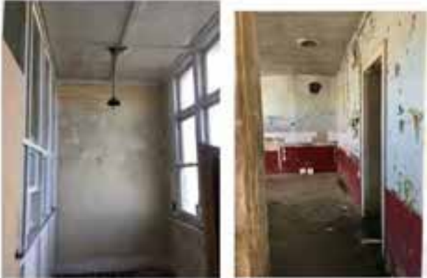
Figure D13. Area D. Typical views of the asbestos clad ceiling and walls of the interior of the 1931 offices.
