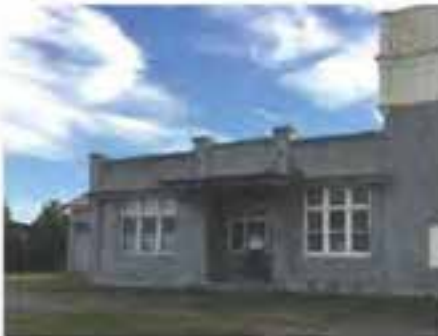
Figure D12. Area D. The south elevation of the 1931 office building. Constructed of brick and rendered, it is divided into three bays with banks of three windows either side of a centrally recessed front door accentuated by the cantilevered porch 'supported' by chains attached to the high parapet. The integrity is high however the architectural design is unremarkable compared with the 1908-09 building.
