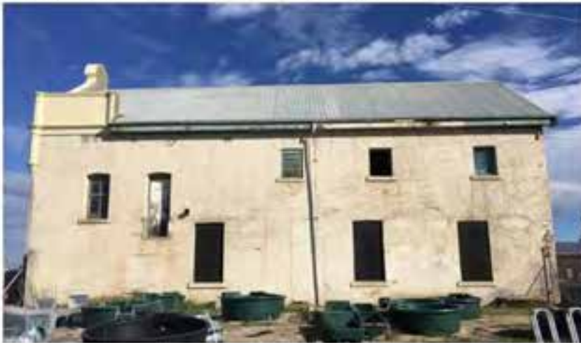
Figure D3. Blue areas A, B, H, I, J. The east elevation has a good degree of integrity. Figure D3 shows the gabled roof clad in galvanised iron and the red brick wall 'bagged'. Segmentally arched openings are located towards the front section. The first floor left hand window is original, the next one has been altered to be a doorway. Two small windows have been bricked up. Towards the northern end of the wall, at first floor level, are three square openings with flat arches, one of which has timber louvres and it is likely that they all had louvres. At ground level are three large flat arched window openings which have been temporarily blocked up on the inside and one that has been infilled. All the openings, except the altered doorway, have projecting sills as seen on the south facade and all of these openings date from 1908-09. The spouting has corroded and is allowing water to soak around the base of the building, most likely contributing to the uneven settling and minor cracking.
