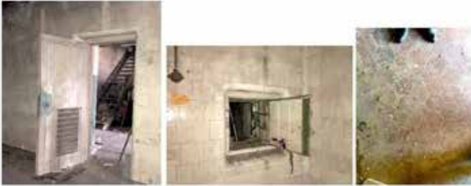
Figure D6. Area A. Detail of door to Area E/E, small hatch and door to Area C, and floor tiles. Note the white glazed tiles with specially curved ones used to cover the edges of the openings and the thick doors on both sides of the small opening.
