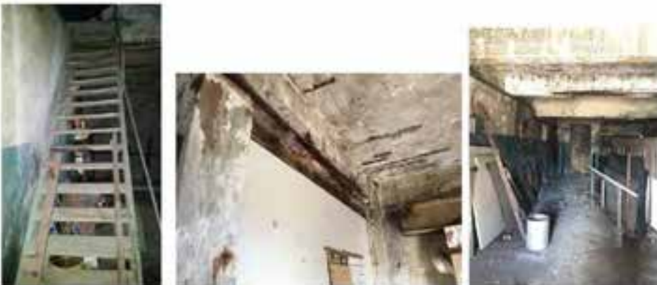
Figure D15. Areas E and F. c1931 building located behind the 1931 office building. The timber staircase, located in AREA E goes to the first floor in AREA K. The other two views are of AREA F.
