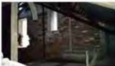
Figure D16, Area K. View towards a former window which has been crudely made into a doorway from Area K into Area H. Source. Andrew Martin 2017.
