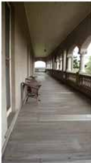
Figure D10. Looking east under the segmental arch, towards the front gates on Settlement Road, showing the unpainted 'ashlar' rendered walls, timber floor of the grand first floor balcony, balustrade and columns. (2011)
