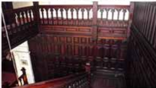
Figure D14. View of fine timber work of the stairs, walls, balustrade, and banister. (2011)
