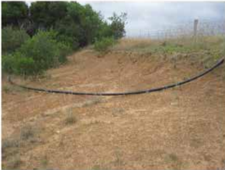
Figure 7: Erosion Embankment (in foreground)
