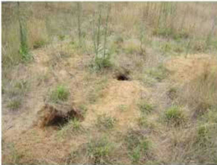
Figure 5: Burrowing in Embankment
